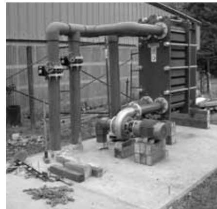
The heat exchanger at Crystal Lake, before completion of the building that protects it.
