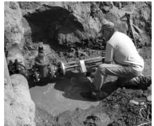
Guy Sparks from Seattle "hot-tapped" water pipes—the least risky method of retrofitting the system.
